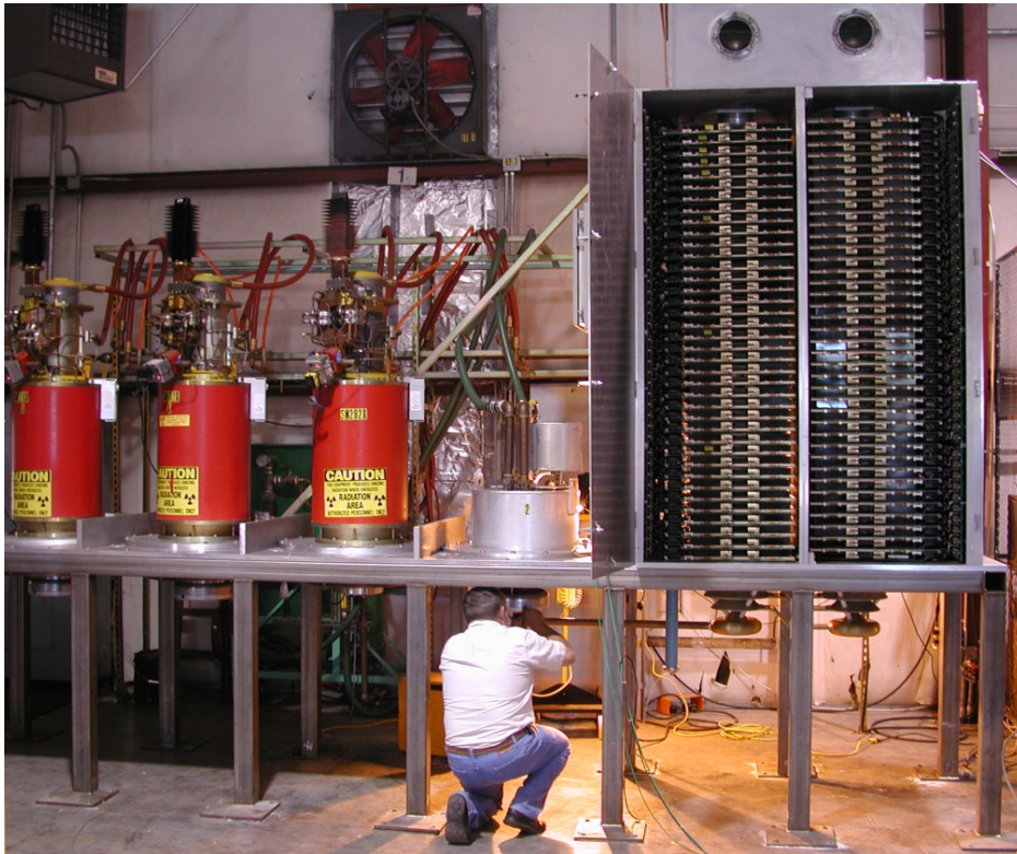
3 turn Secondary with water load
